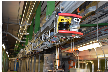
Figure 4: Train Inspection Monorail which can haul specialized wagons i.e. with a manipulator.
