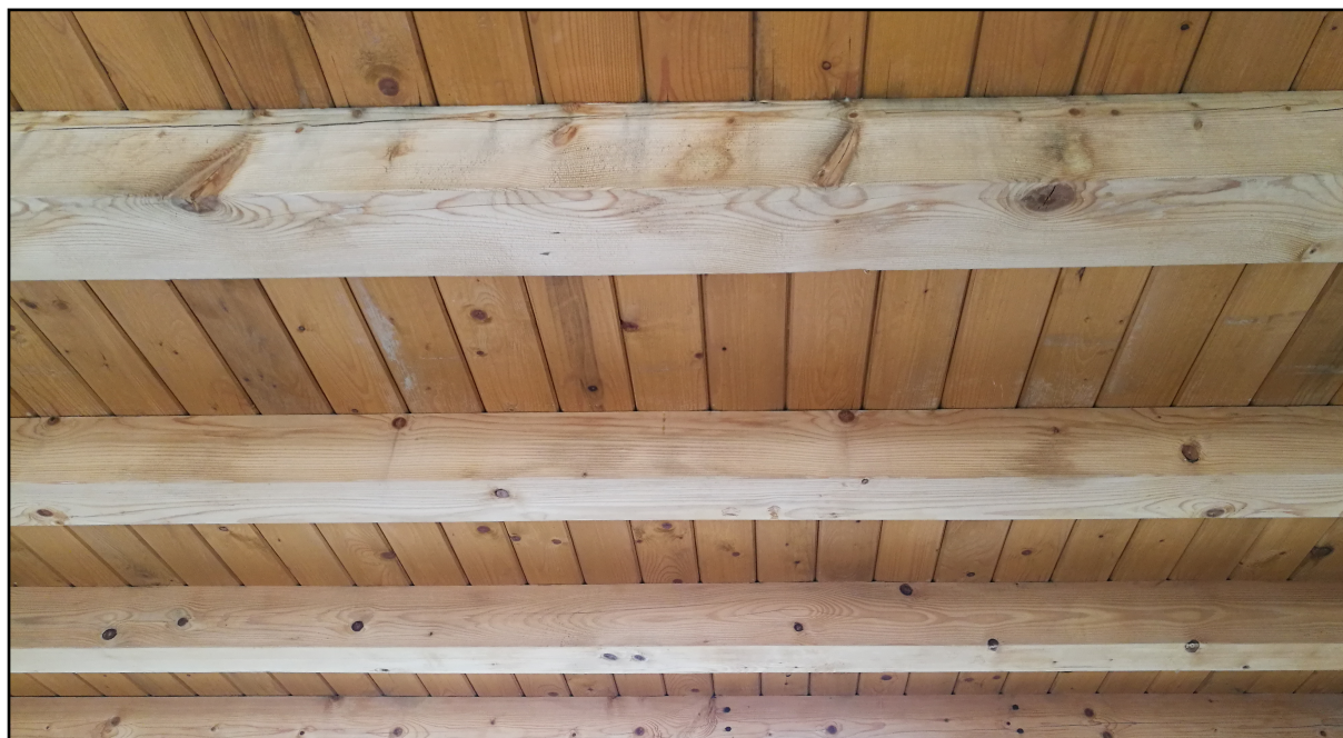
Figure 9 - Photograph of the different sizes of wood used in the structure of buildings
