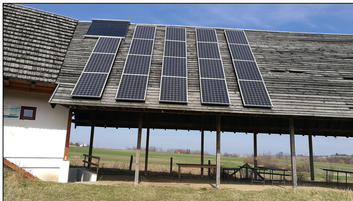
Figure 6 - Photograph of a portion of installed solar panels
