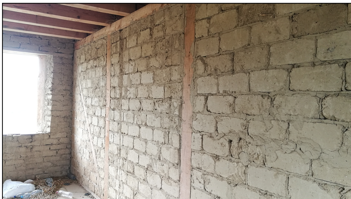
Figure 11 - Photograph of the wall inside the homes
