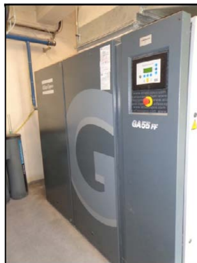
Figure 4.6 Compressor from dry milling department
