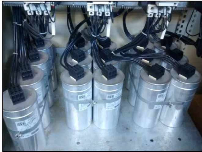
Figure 4.2 Capacitor's battery inside of the transformer
