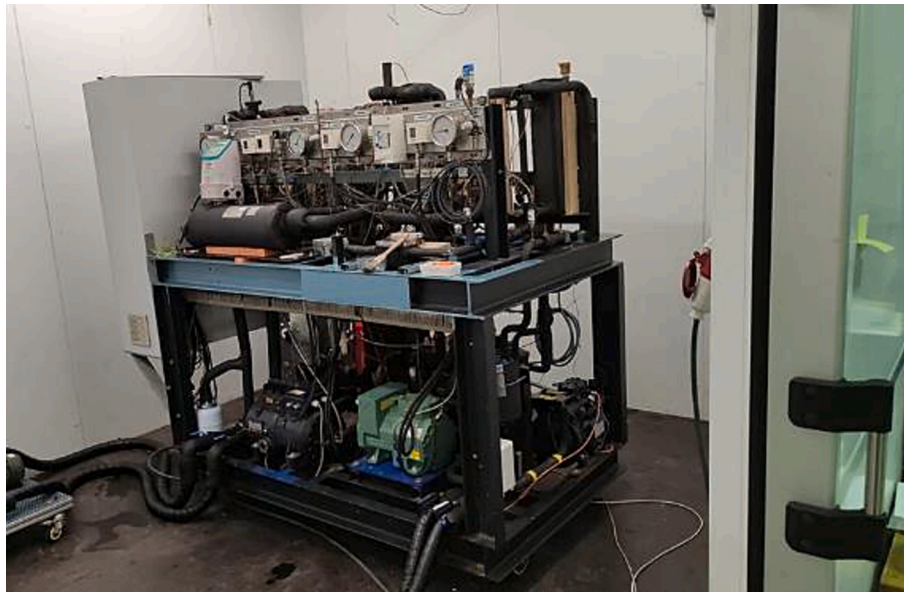
Fig. 3. General view of the experimental cascade refrigeration plant.
