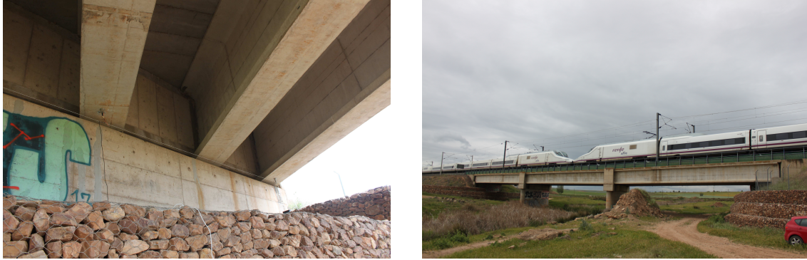
Figure 1: Jabalón Bridge: detail of the girder deck and end diaphragms and general view.
