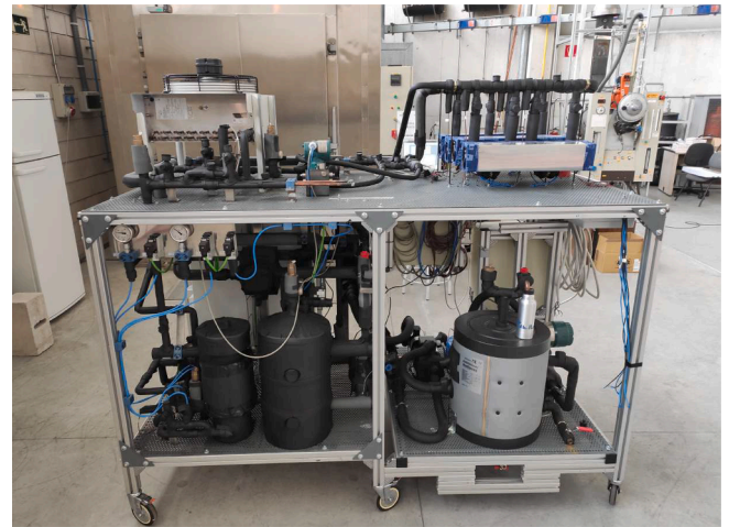
Fig. 2. Experimental refrigeration facility.
