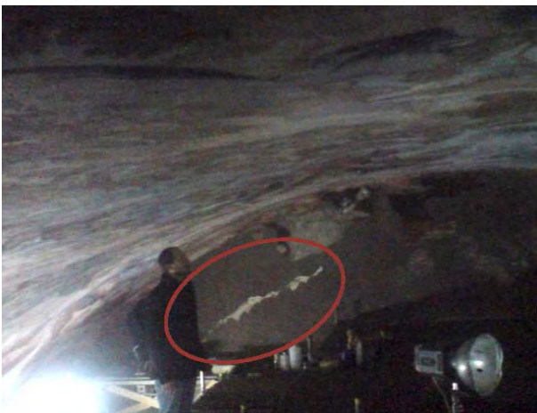
Figure 25. Interior façade view. Crack
