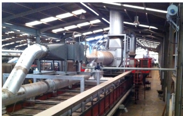
Fig. 2. Thermal oil facility
