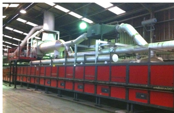
Fig. 1. Heat exchanger integrated in furnace chimney
