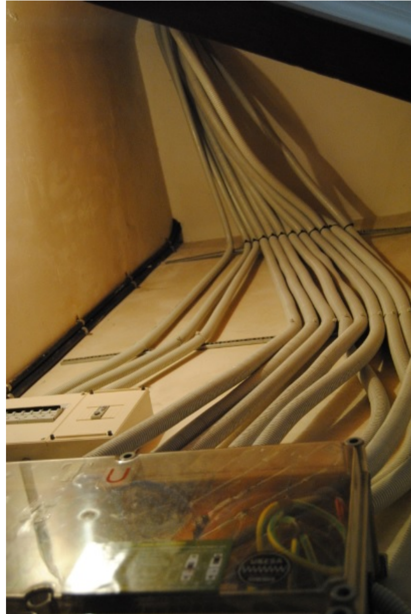
Suministro electrico. Red. [Ref. IN006]
