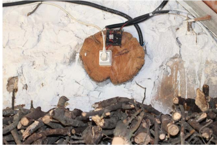
Figure7. State of the installation.
