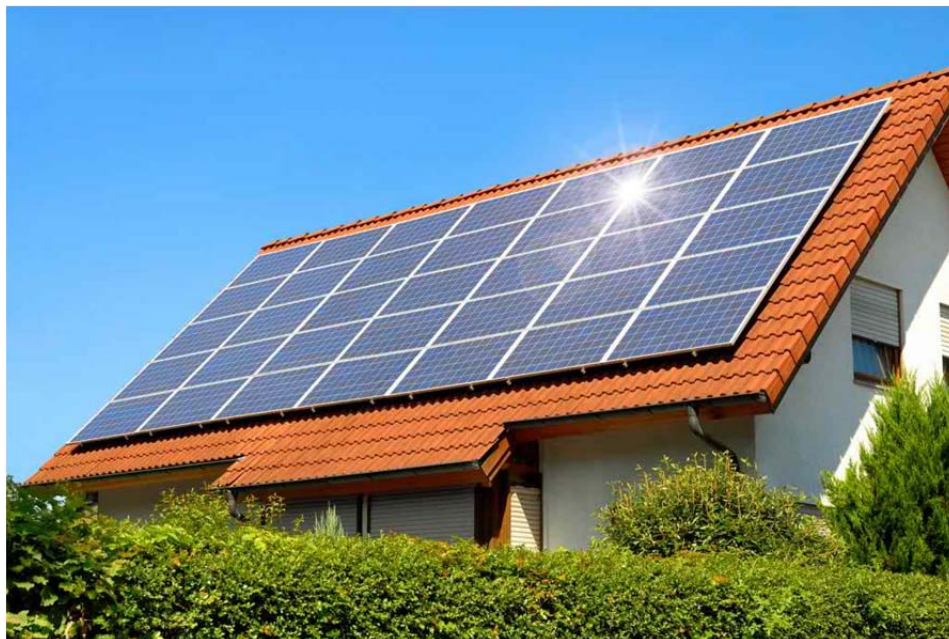
Figure 8. Roof - photovoltaic system
