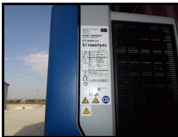
Figure 26. Inverter technical information
