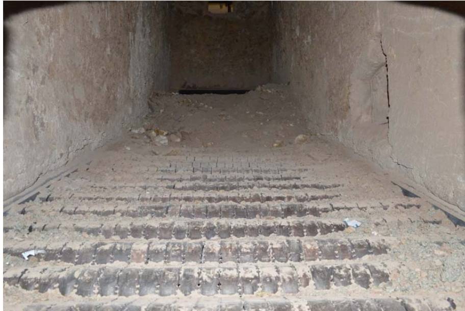
Figure 7. Inside the boiler
