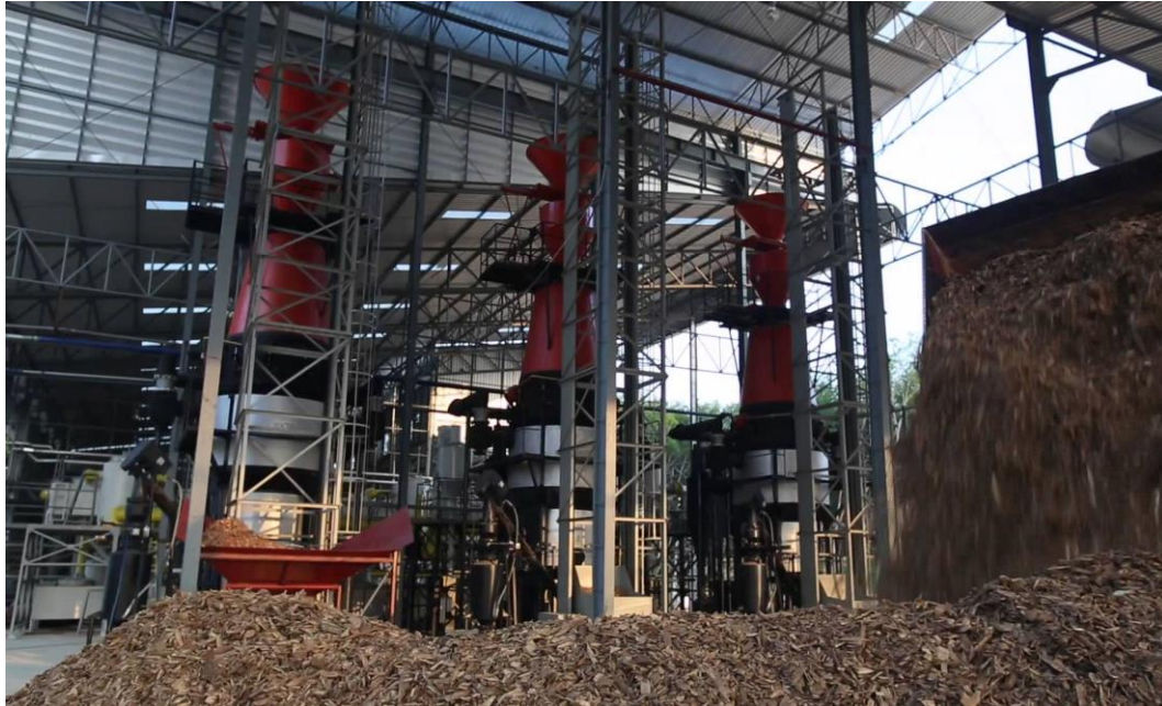
Figure 12. Biomass Gasification Power Plant - Sustainable Way.
