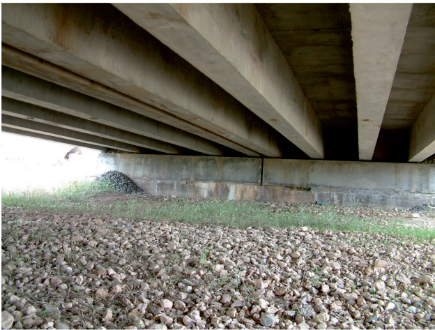
Figure 1: Railway bridges in Spanish lines composed by simply-supported bays of short-to-medium span
