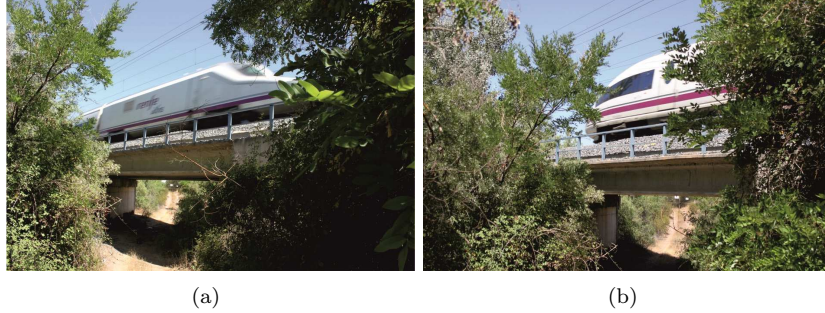
Figure 10: Arroyo Bracea I Bridge. Experimental campaign images: (a) RENFE Class 102 (Talgo 350) train passage at v = 263 km/h and (b) RENFE Class 103 (ICE 3) train passage at v = 279 km/h.
