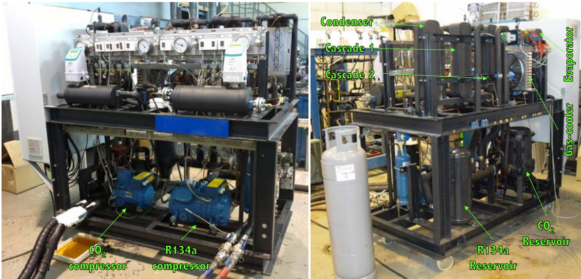
Figure 2. View of the cascade refrigeration plant
