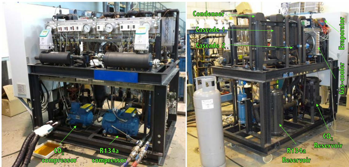
Figure 2. View of the cascade refrigeration plant.
