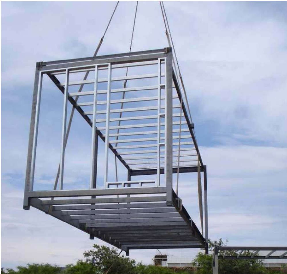
Ilustración 17 Main structural frame made in rolled steel, together with galvanized steel frame in the walls' substructure; Fuente: eBRICKhouse project manual
